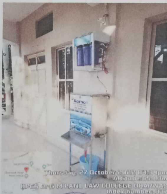
Purified Drinking Water facility for Students.
